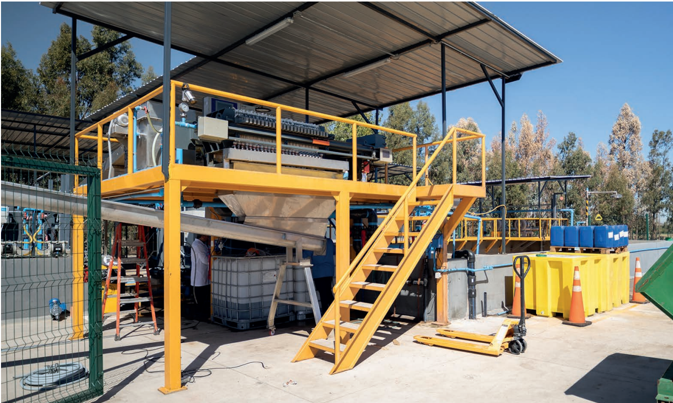
Depuradora de la planta de producción Fruselva Chile. / Wastewater treatment plant at the Fruselva production facility in Chile.
